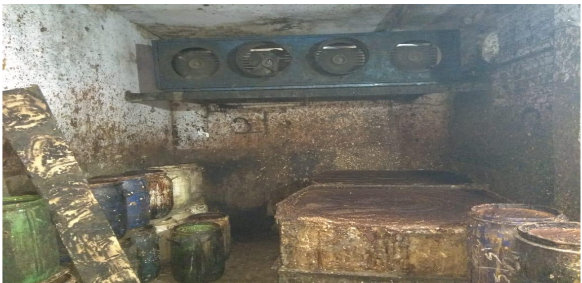
Pic 18: Concentrating process through evaporator
